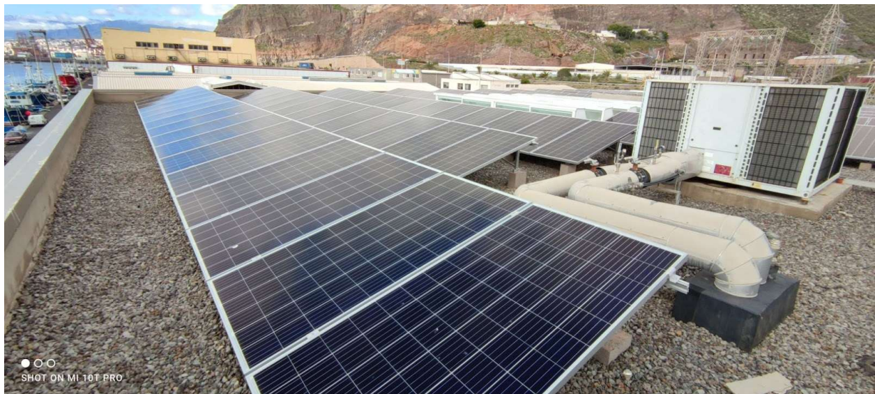
Image 2. Photovoltaic installation of Fish Market
