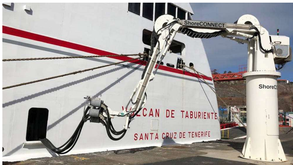
Image 1. Vessel connected to the OPS in La Gomera port.
